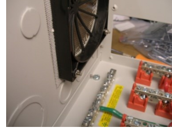
E-Panel earth ground bus (AC & DC)
